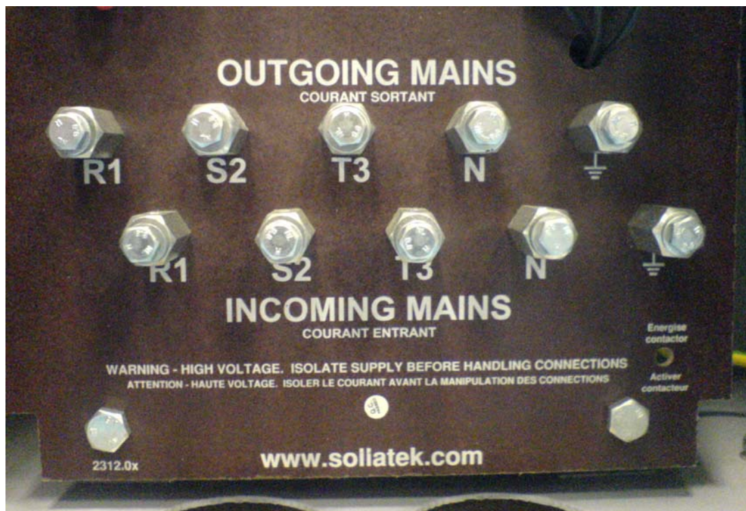
Photo 2.6.1 Typical Terminal Arrangement
